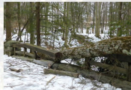
Oak tree damages bridge
