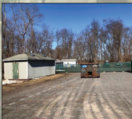
Construction on the maintenance area in the overflow parking lot began in February.
